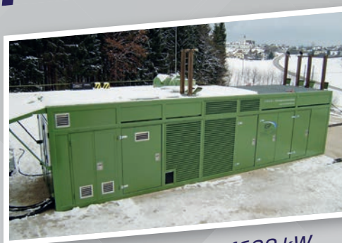
Mobiles Dieselaggregat 1600 kW
